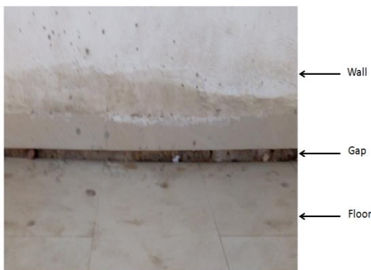
Fig. 1: Gap Between the Wall and Floor of a Building in the University
