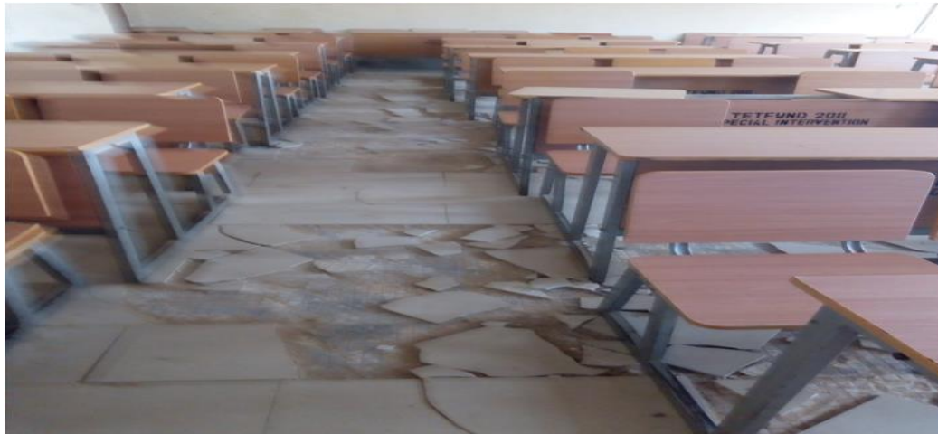
Fig. 3: Floor Cracking in a Classroom in the University
